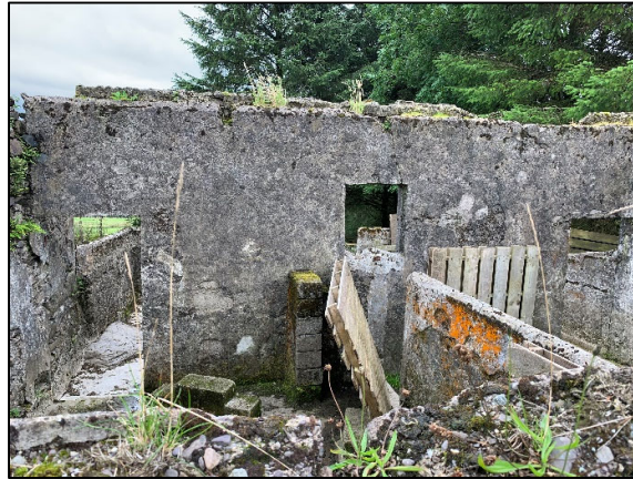
Plate 3-1: Example of derelict buildings present at Inchamore
