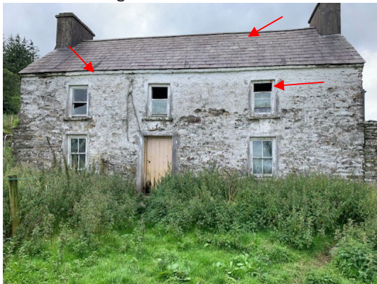
3. Derelict dwelling indicating potential access points via soffit, ridge tiles and gaps in roof tiles and open window.
